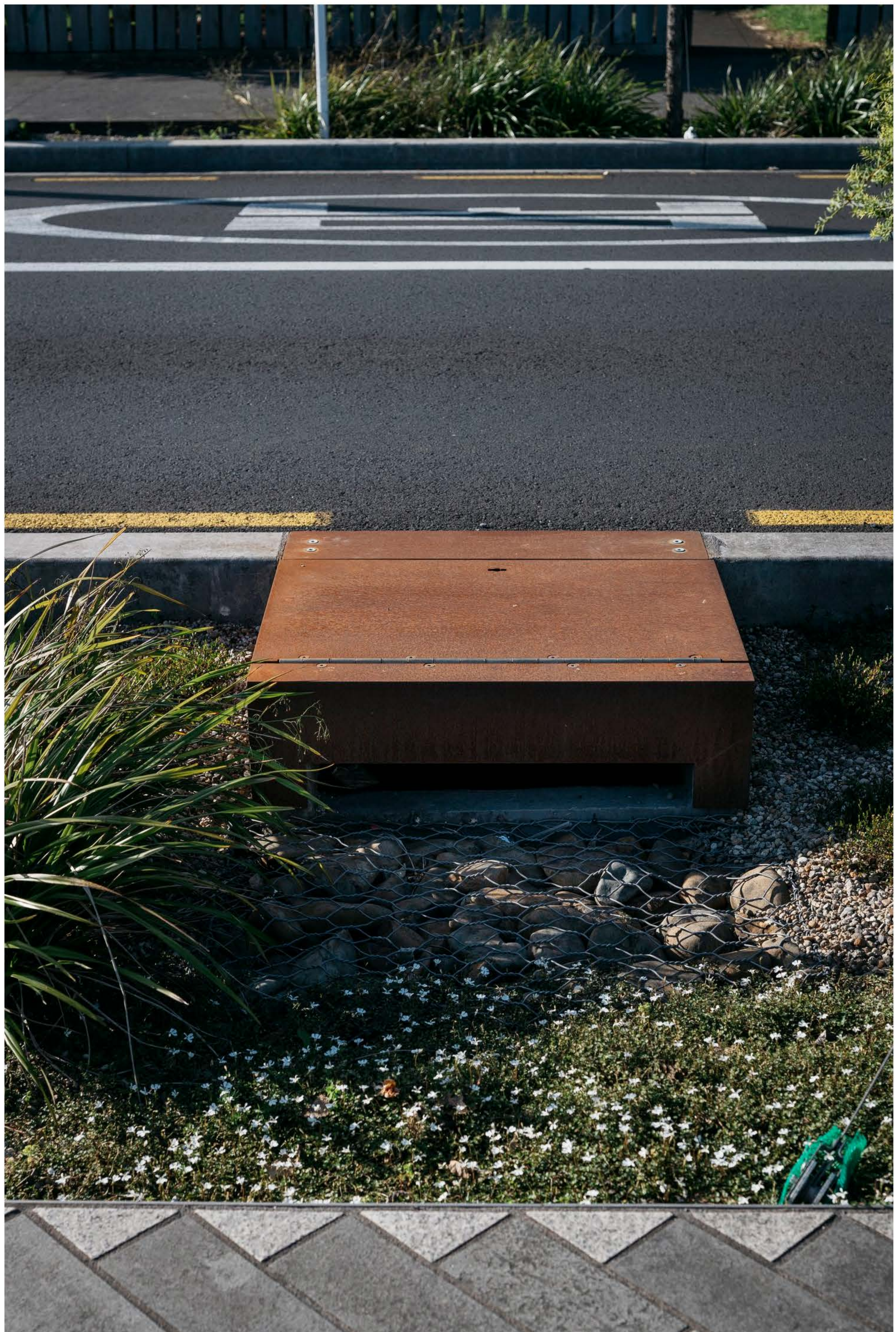
The Boffa Miskell team developed an improved bio-filtration garden forebay design to filter floating rubbish and sediment from incoming water from the road before reaching the garden.
